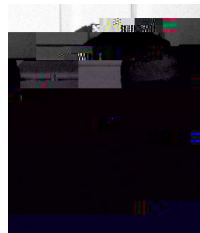
JAY LOFTON TEAM R4 07-18-21 AIR COMPRESSOR
